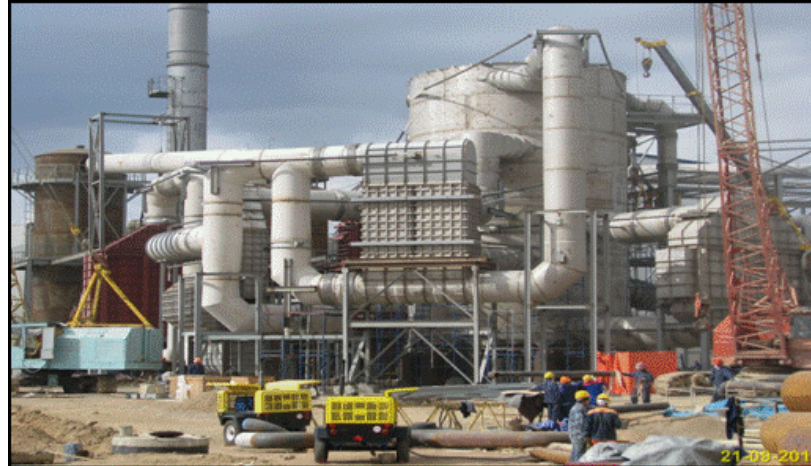
SKZ-U Converter 80% Complete
