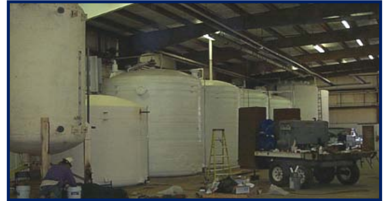
Irigaray Central Processing Facility
