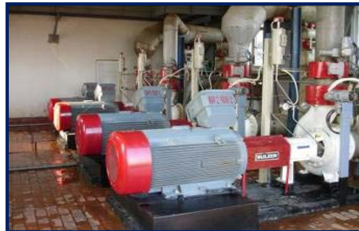
Pump House at Akdala
