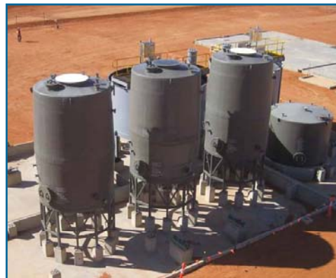
Honeymoon – Precipitation tanks
