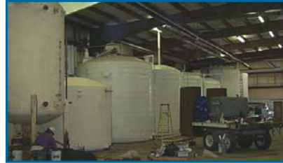
Irigaray Central Processing Facility
