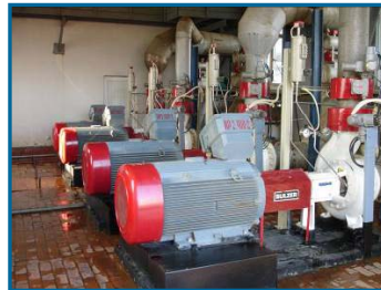
Pump House at Akdala
